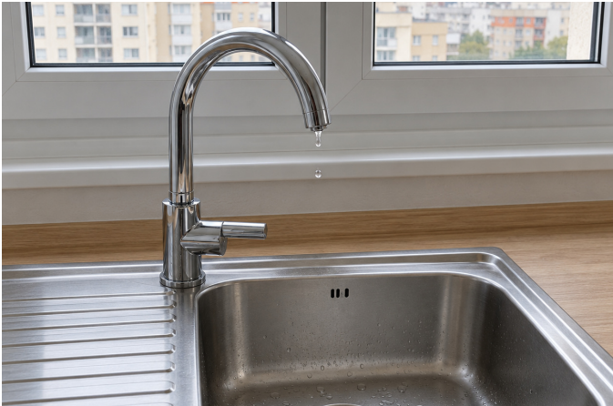
F17 Mutfak - batarya
